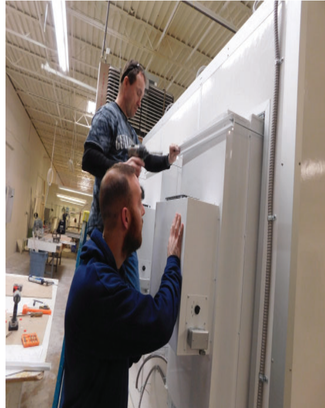
Installed (HEPA Filtration unit D).
