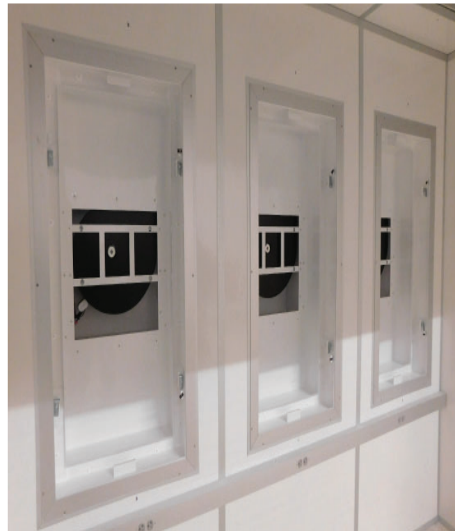
Interior view of HEPA filtration back wall.
