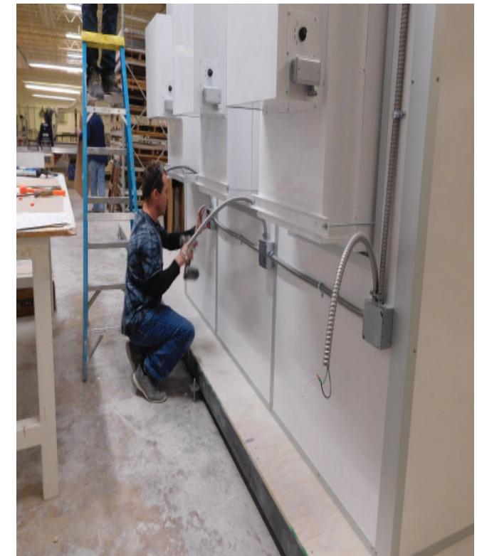
Note: back view of conduit connections.
