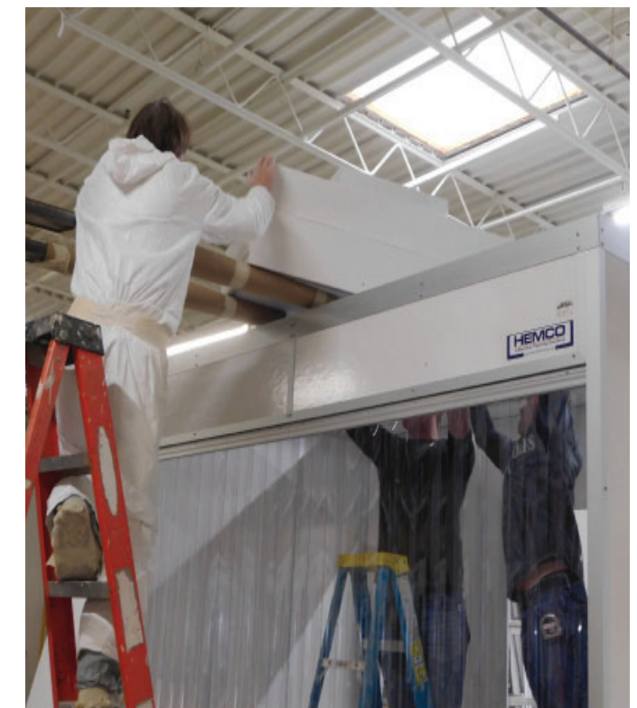
Install (HEPA Filtration unit B) using a forklift to move it into place
