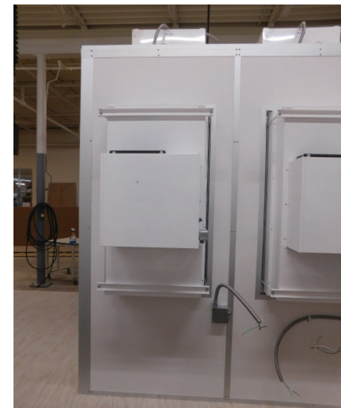
Installed (HEPA Filtration unit B).
