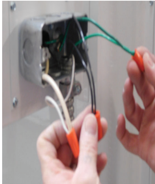
Note: Electrical Box on back of HEPA filtration unit located on back.
