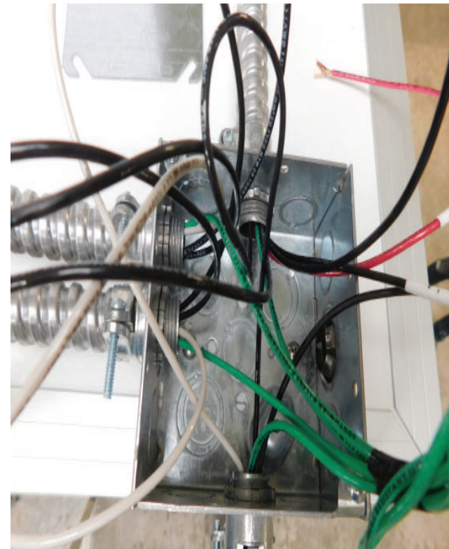
Note: Electrical Box on top of Hood located on back left corner.
