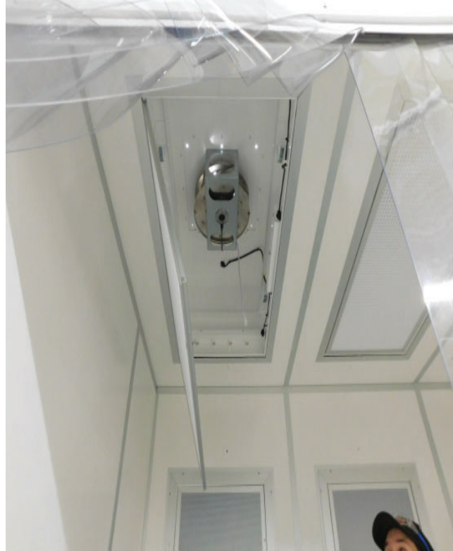
Interior view of HEPA filtration ceiling
