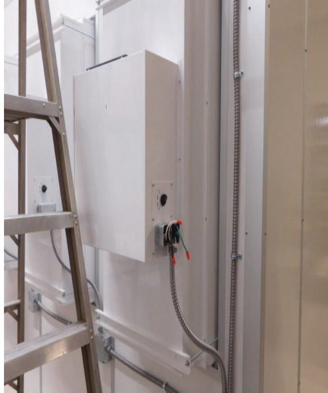
Note: Electrical Box on back of HEPA filtration unit located on back.
