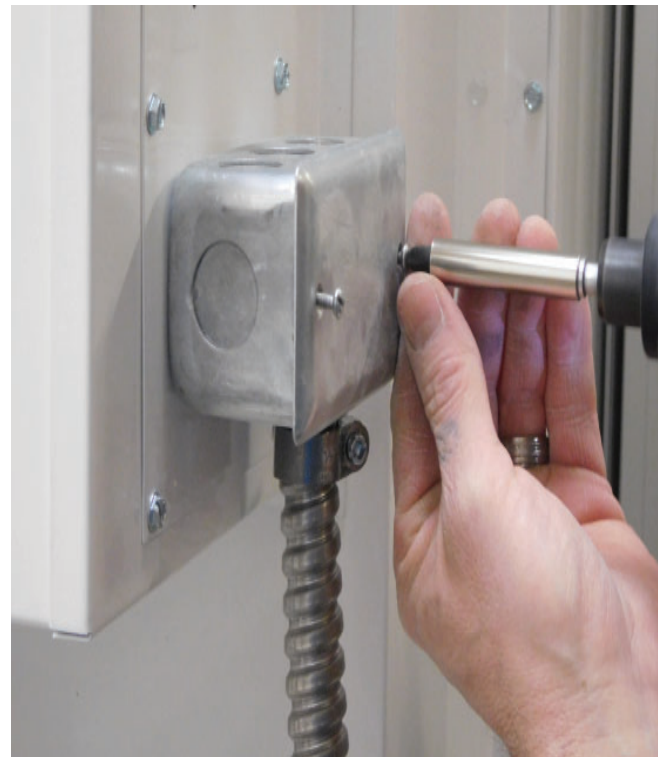
Secure cover on junction box.
