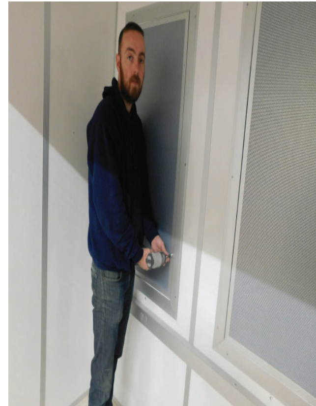
Mount prefilter covers for HEPA filtration back wall on inside.
